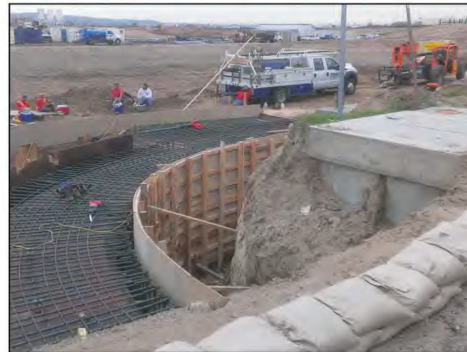
After discovery of toxic contamination while constructing this storm drain at the Portola High School site in November of 2014, the City's environmental consultant reported that he expected DTSC to immediately order new testing for toxic petrochemicals. The expected testing never happened.
